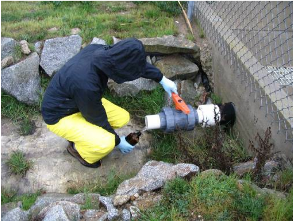
Figure 1. Stormwater discharges to the slot drain and is conveyed offsite through a valved pipe.
