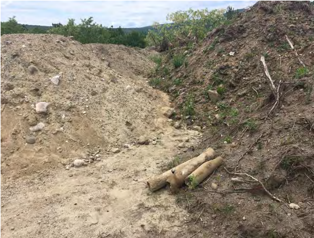
View of the three pieces of possibly asbestos-containing pipe pulled from the 10 dump truck loads of sandy gravel fill and set aside.
