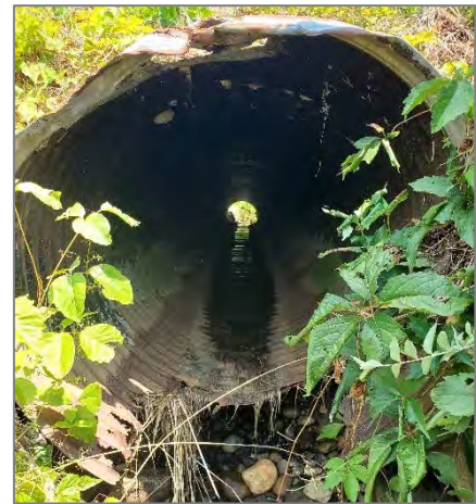
Example of a corrugated metal culvert in deteriorated, poor condition. (CEI photo)
