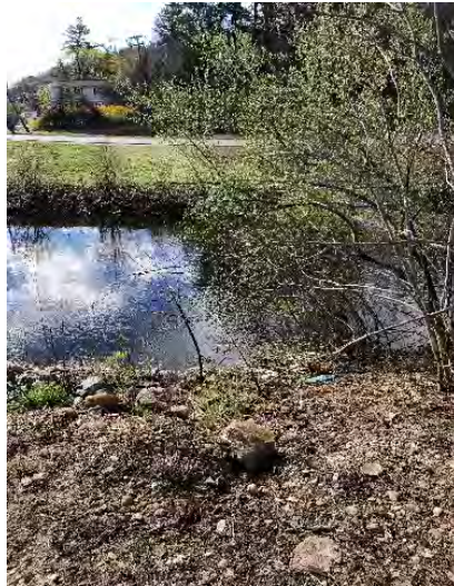
Photo 3-2: Loose stone and sand on slope.
