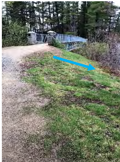
Photo 4-3: Lack of defined edge of dirt path allows for runoff to enter grassed area.
