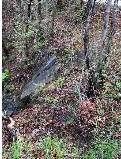
Photo 16-2: Steep stream embankment.
