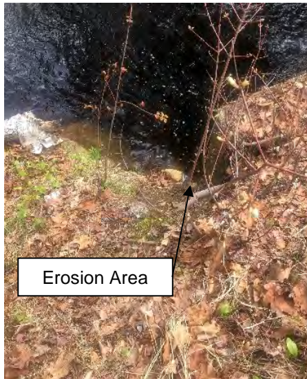
Photo 12-1: Erosion on the edge of wingwalls.
