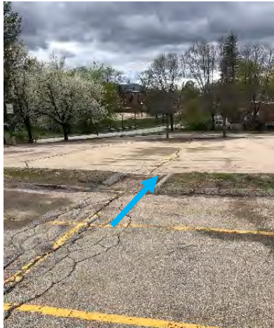
Photo 8-1: Parking lot area with cracks in pavement.
