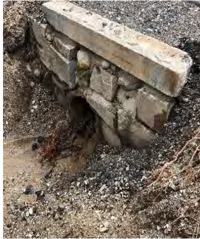
Photo 10-2: Drainage outfall/headwall in need of repair.
