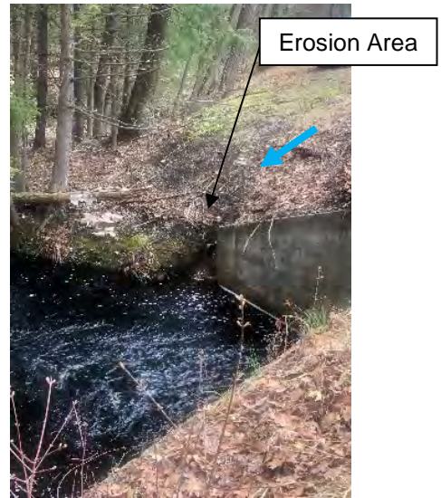
Photo 12-3: Erosion on the edge of wingwalls.
