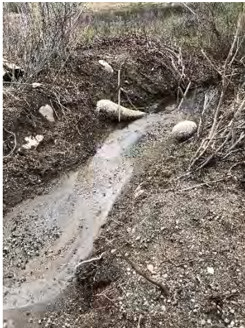
Photo 10-1: Sediment buildup downstream of outfall.
