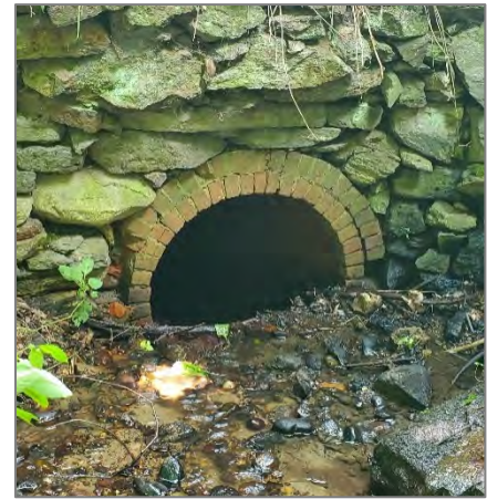
Example of an undersized culvert prone to clogging with sediment and debris. (CEI photo)
