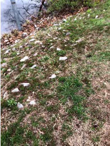
Photo 4-5: Riprap area in need of additional riprap to prevent future erosion.
