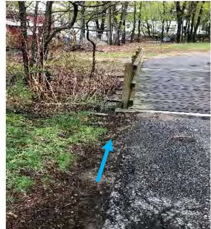
Photo 8-3: Erosion from walking path down to brook.
