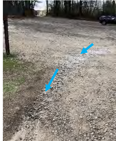
Photo 1-3: Dirt parking area eroding and washing into pond.
