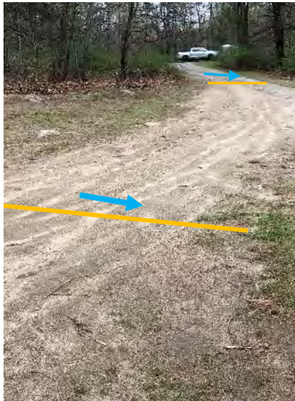
Photo 5-1: Dirt road with signs of erosion.
