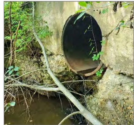
Example of a perched culvert that prohibits upstream aquatic organism passage. (CEI photo)
