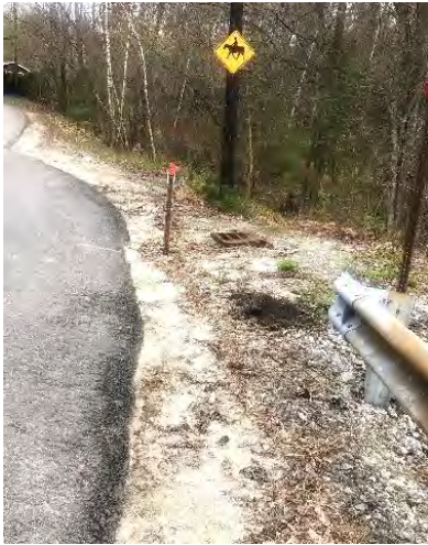
Photo 13-1: Edge of Grapevine Rd.
