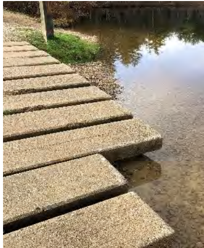
Photo 1-2: Concrete block boat ramp undercut.
