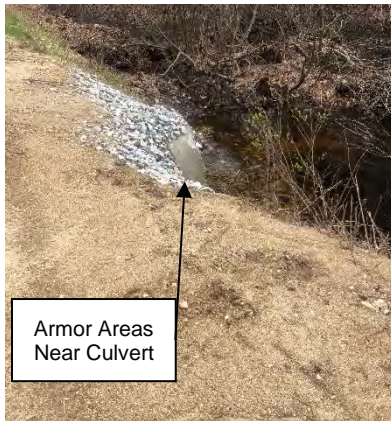
Photo 14-1: Loose sandy soils observed near culvert inlet.
