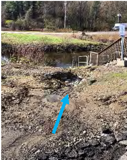
Photo 3-1: Severe erosion adjacent to water access point.
