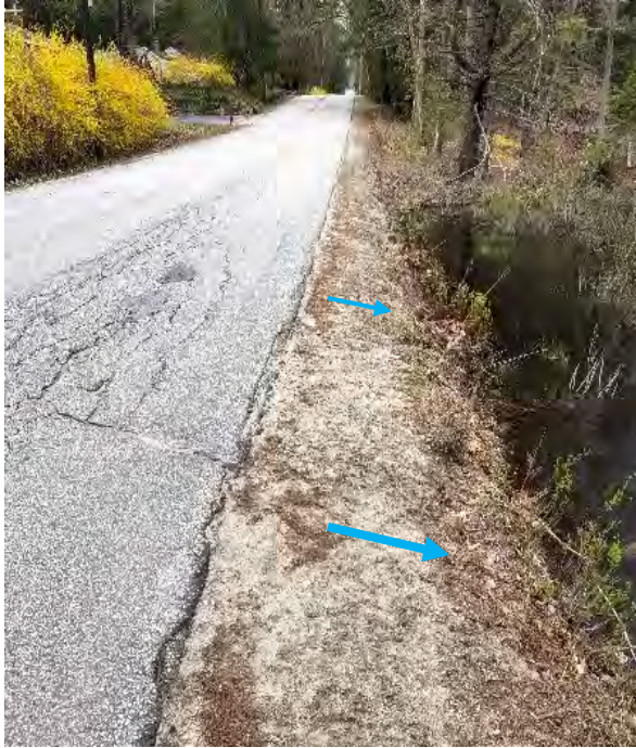
Photo 11-1: Direct runoff into Boutwell Mill Brook.
