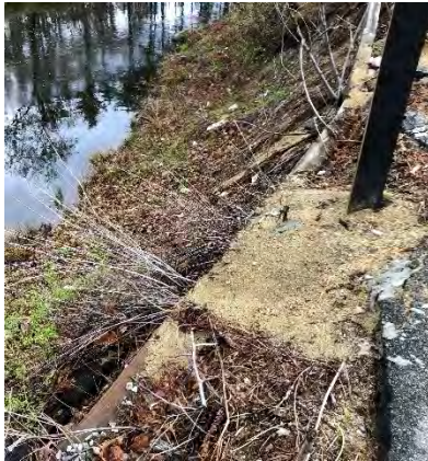
Photo 15-1: Edge of parking lot and steep slope with obvious signs of erosion.
