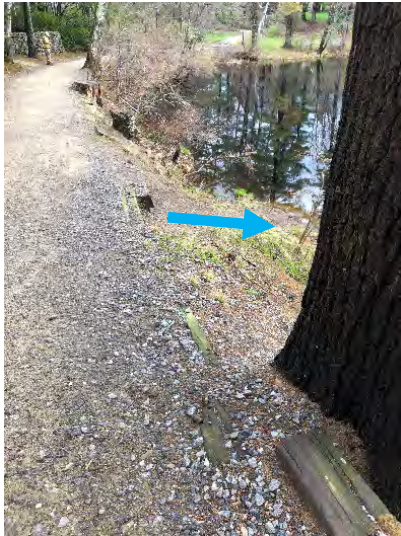
Photo 4-11: Shoreline erosion and lack of vegetated buffer.
