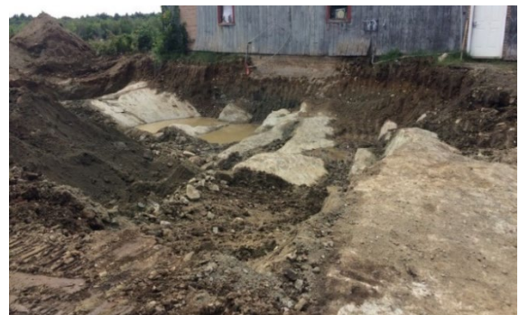
These photos show the contaminated soil being excavated. Note: In the picture at the bottom, you can see that the excavation extended to the uneven bedrock surface
