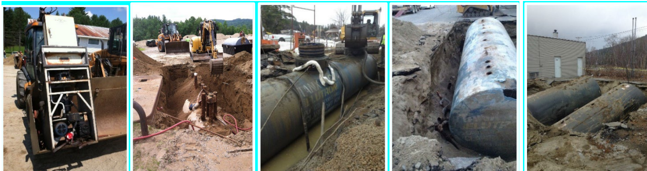
Images below feature, from left to right: a 50' vintage dispenser, post removal; a tank top uncovered during UST removal; a Tank that was buried under the water table after controlled float out of the excavation; USTs prior to removal from tank graves.
