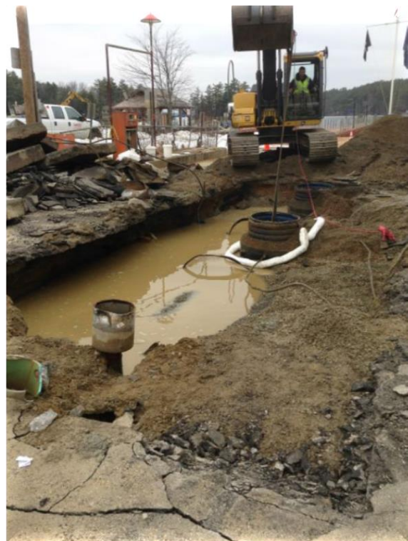
Submerged Marine Patrol Tank exposed for removal. The hold down straps were broken, and the tank was floated so that water would not get in the tank during cleaning.
