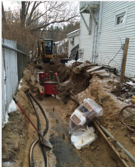
Tank being removed from a tight alley in Gilford. Tanks had to be dragged out and around the back due to power lines and other obstructions.
