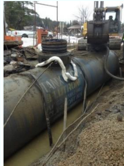
Tank that was buried under the water table after controlled float out of the excavation.
