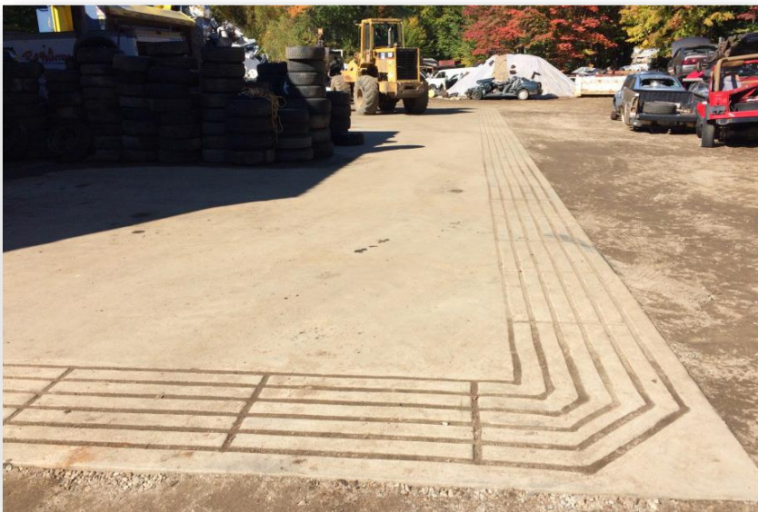
A concrete spill-prevention pad installed by the program. Note the positive limiting barrier (PLB) in the photo. The PBL consists of grooves in the concrete designed to trap spills until they can be cleaned up.
