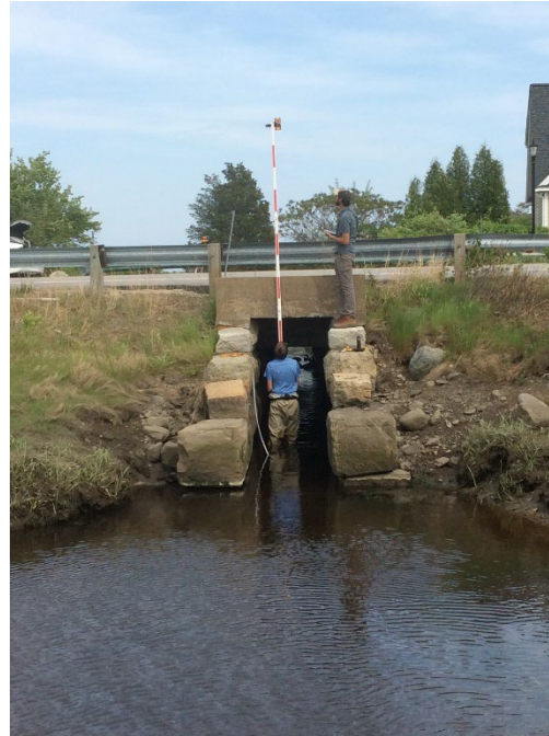
Figure 2. Culvert inlet at Route 1A and an unnamed tributary of the Awcomin Salt Marsh.
