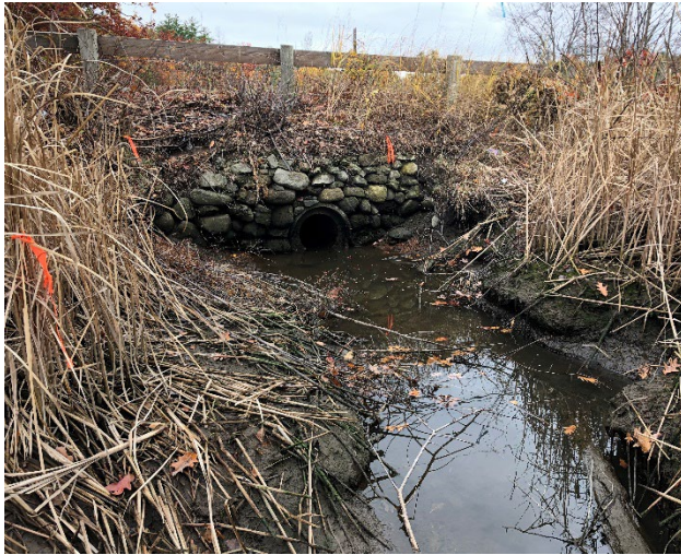
Figure 3. Culvert inlet at Squamscott Road and an unnamed tidal tributary of the Chapman’s Landing Salt Marsh.
