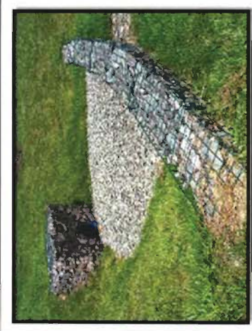
Plunge pool with gabion level spreader
