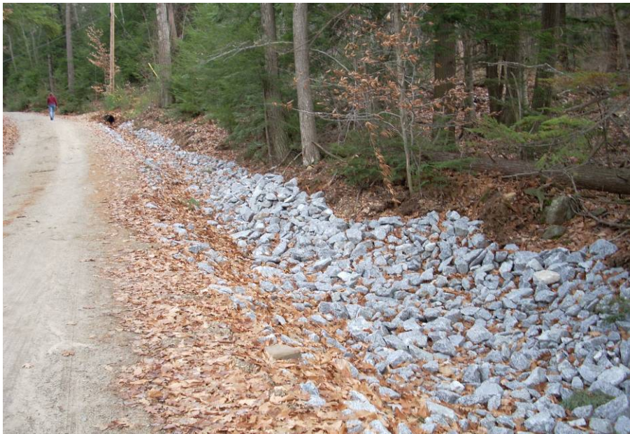
A stone-filled infiltration trench constructed to intercept runoff from the adjacent unpaved road in the Silver Lake watershed (Harrisville, NH).
