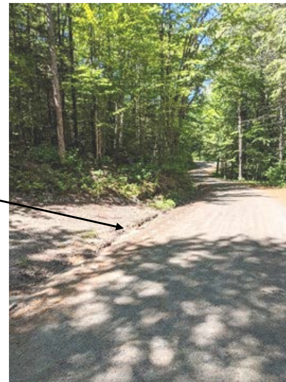
Photo 12-2: Roadside erosion, view looking east
