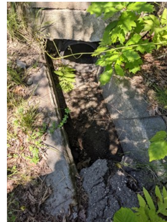
Photo 6-3: Culvert Channel Extension Filled with Sediment
