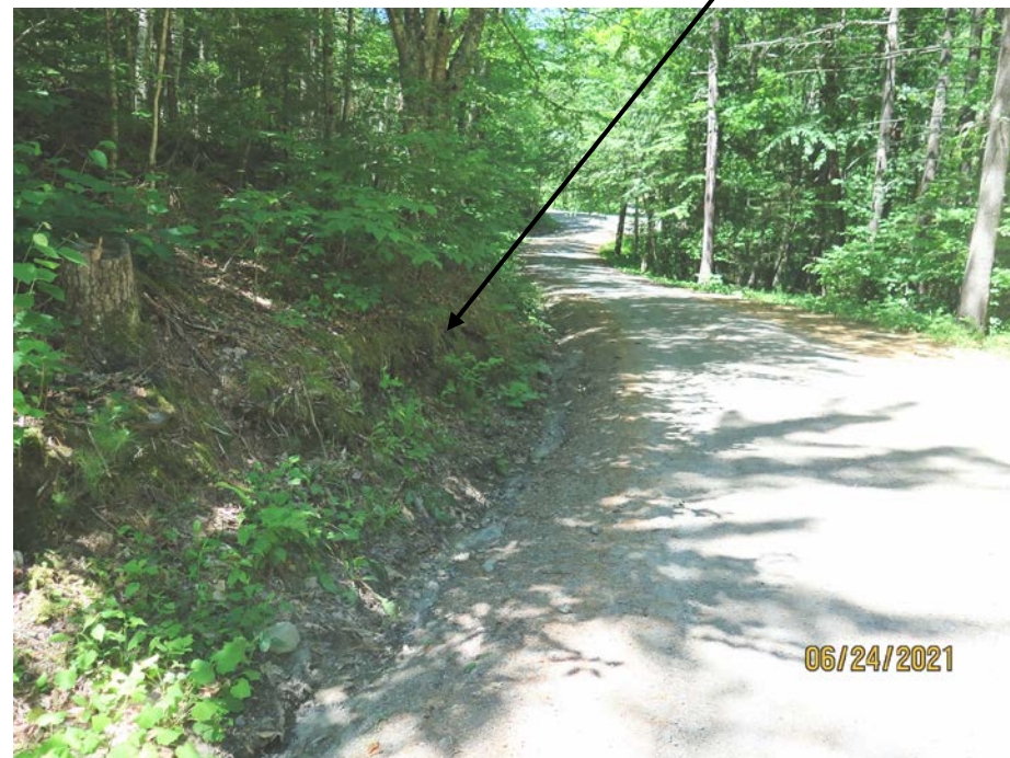
Photo 12-2: Roadside Erosion - Steep Slope
