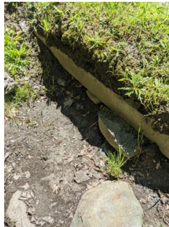
Photo 6-2: Culvert Completely Buried
