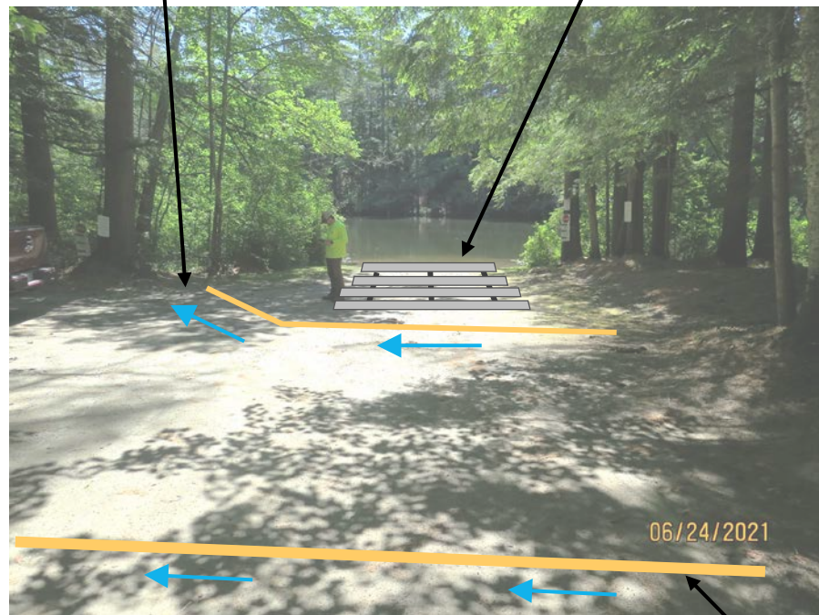
Photo 7-4: Minor boat ramp erosion
