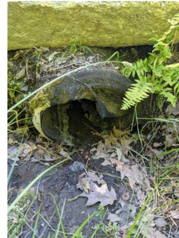
Photo 6-1: Culvert Partially Filled with Sediment
