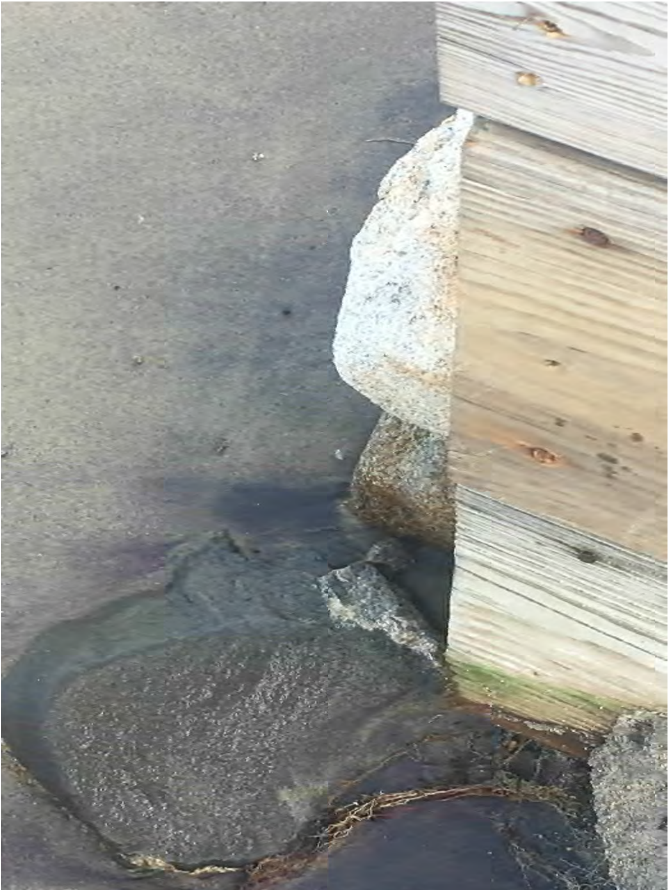
9-1-19 – additional rocks exposed due to erosion.
