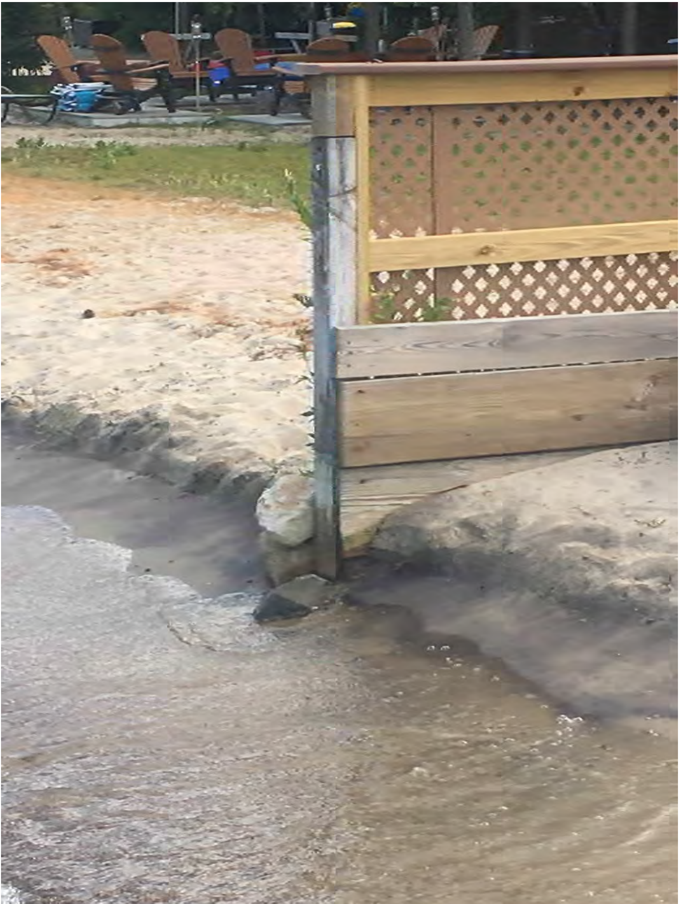
Picture taken 9-1-19 – The water level has done additional erosion (can no longer walk around fence to our neighbors yard without walking in the water).
