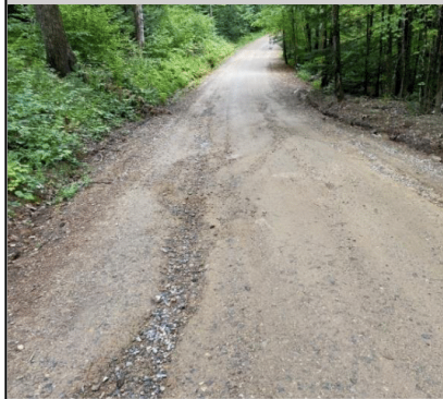
Erosion along Kaulback Road.
