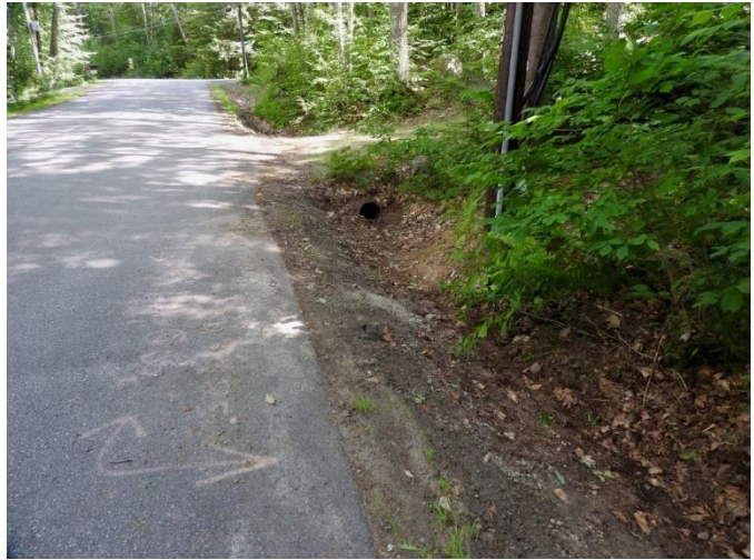
Example of a road ditch with accumulated sediment and vegetation scraped out to maintain hydraulic capacity, as part of the town’s maintenance practices.
