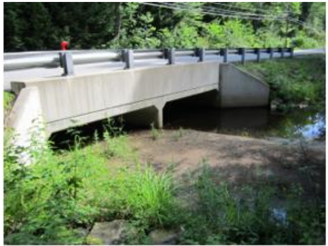
Sedimentation evident at a new box culvert along Black Brook at the Black Brook Rd crossing. Photo courtesy of Lang (2021).
