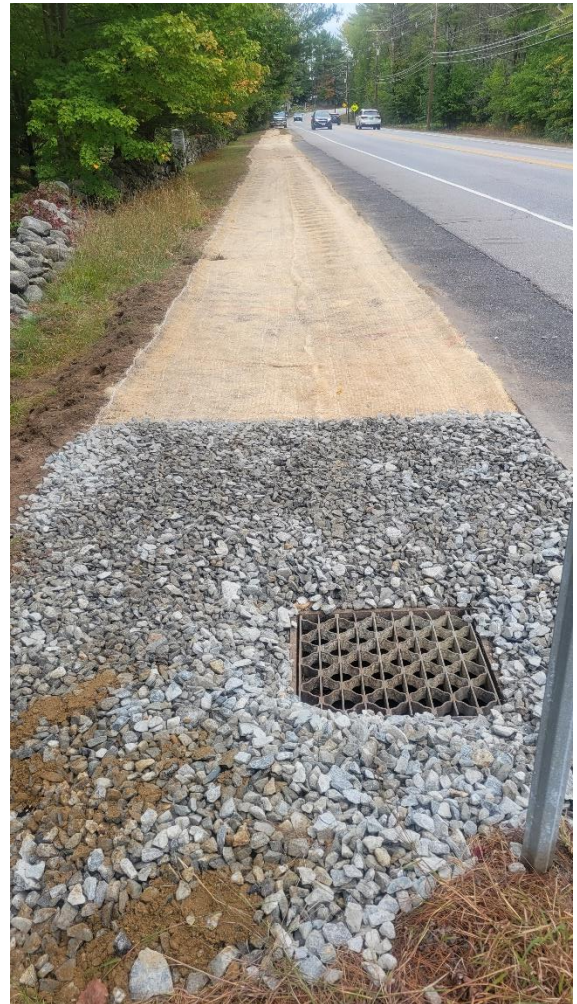
Improved road ditch maintenance along Route 25 in Moultonborough. Photo credit: Kevin Kelly.
