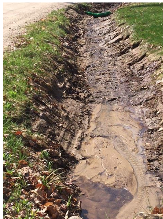
Road ditch maintenance causing erosion on Avon Shores Rd, May 2022. Photo credit: Kevin Kelly.
