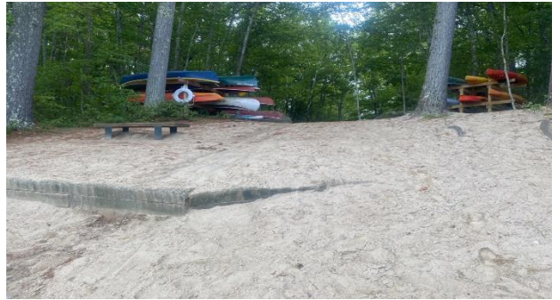
Steep grade leading from parking area directly to pond, showing overtopped, wooden retaining wall.
