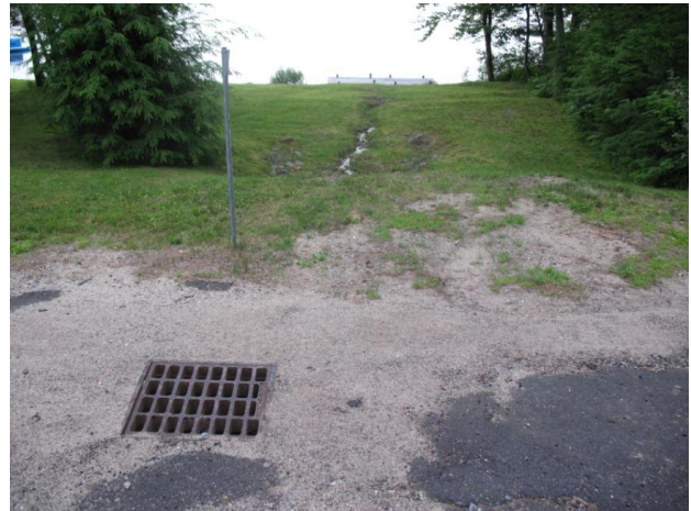
Catch Basin at BMP Site 23
