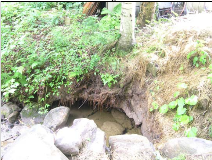
Photo 23: Severe bank erosion at outlet of C19.
