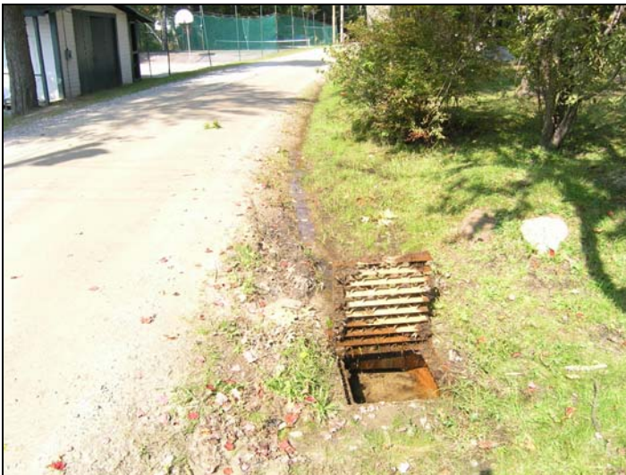
Photo 14: CB7 with sediment.
