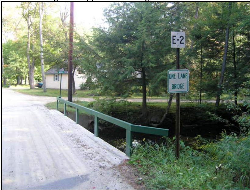
Photo 2: Bridge E-2 decking with sediment along shoulder.
