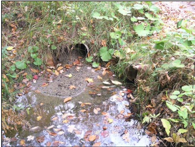
Photo 26: C23 outlet and C24 inlet at house #58
