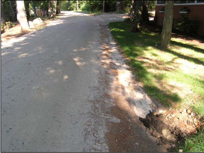
Photo 8: North Shore Road, looking north in front of house #168. CB3 located in bottom right of photo.
