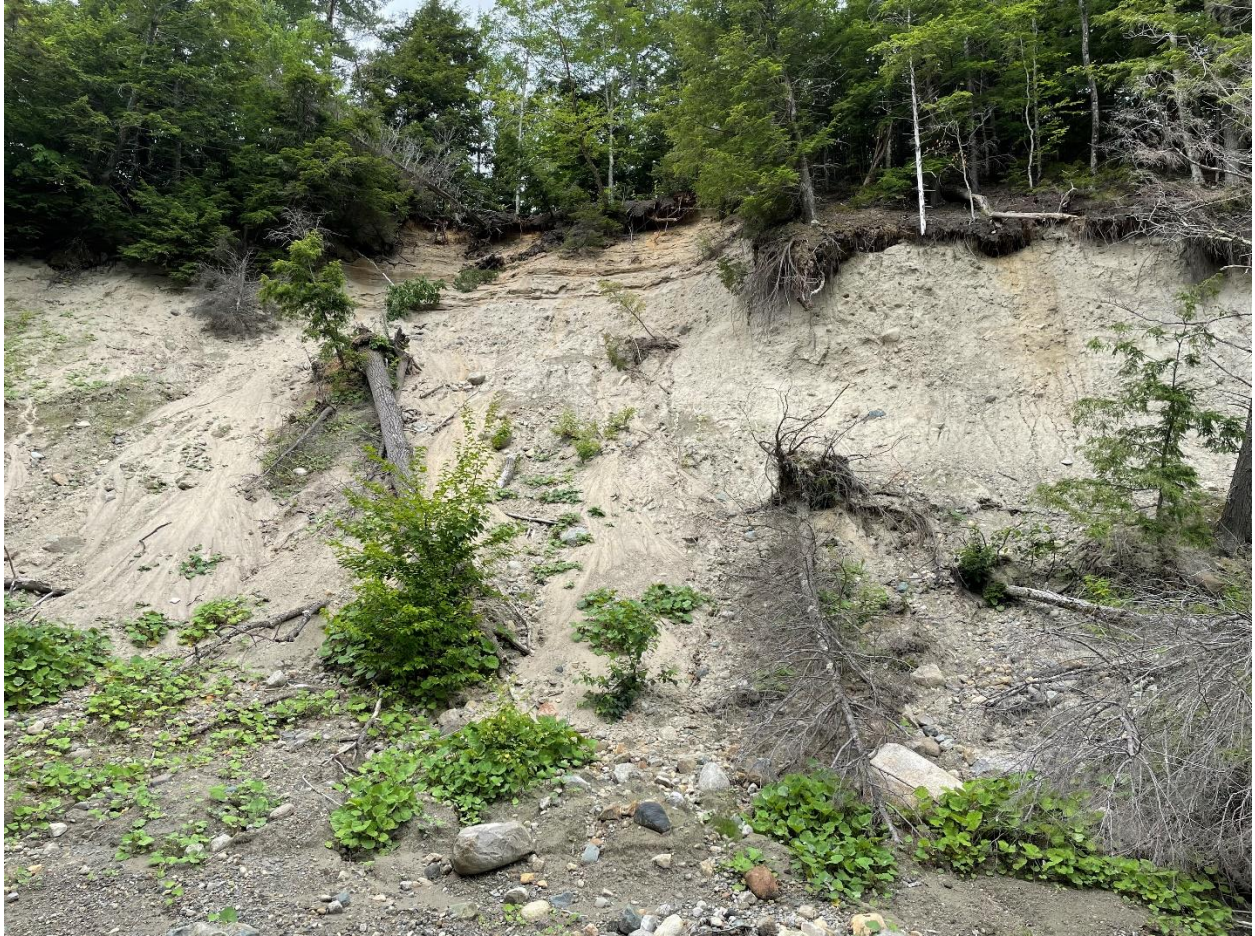
Figure 7. Photograph looking west across Tunnel Brook along U.S. Forest Service Road 162 at 75-foot vertical exposed section of ice-contact stratified sand and gravel interbedded with till on the right and a large block of compact laminated clays at the left that indicates glaciofluvial transport from up valley (1255-ft elevation, 44° 5.10984' N, 71° 49.95804' W).
