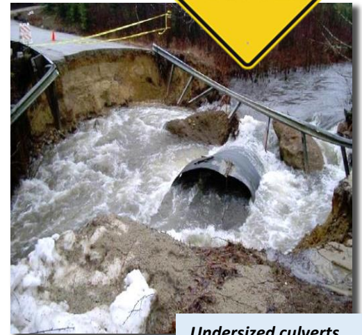
Undersized culverts can cause significant road damage!
