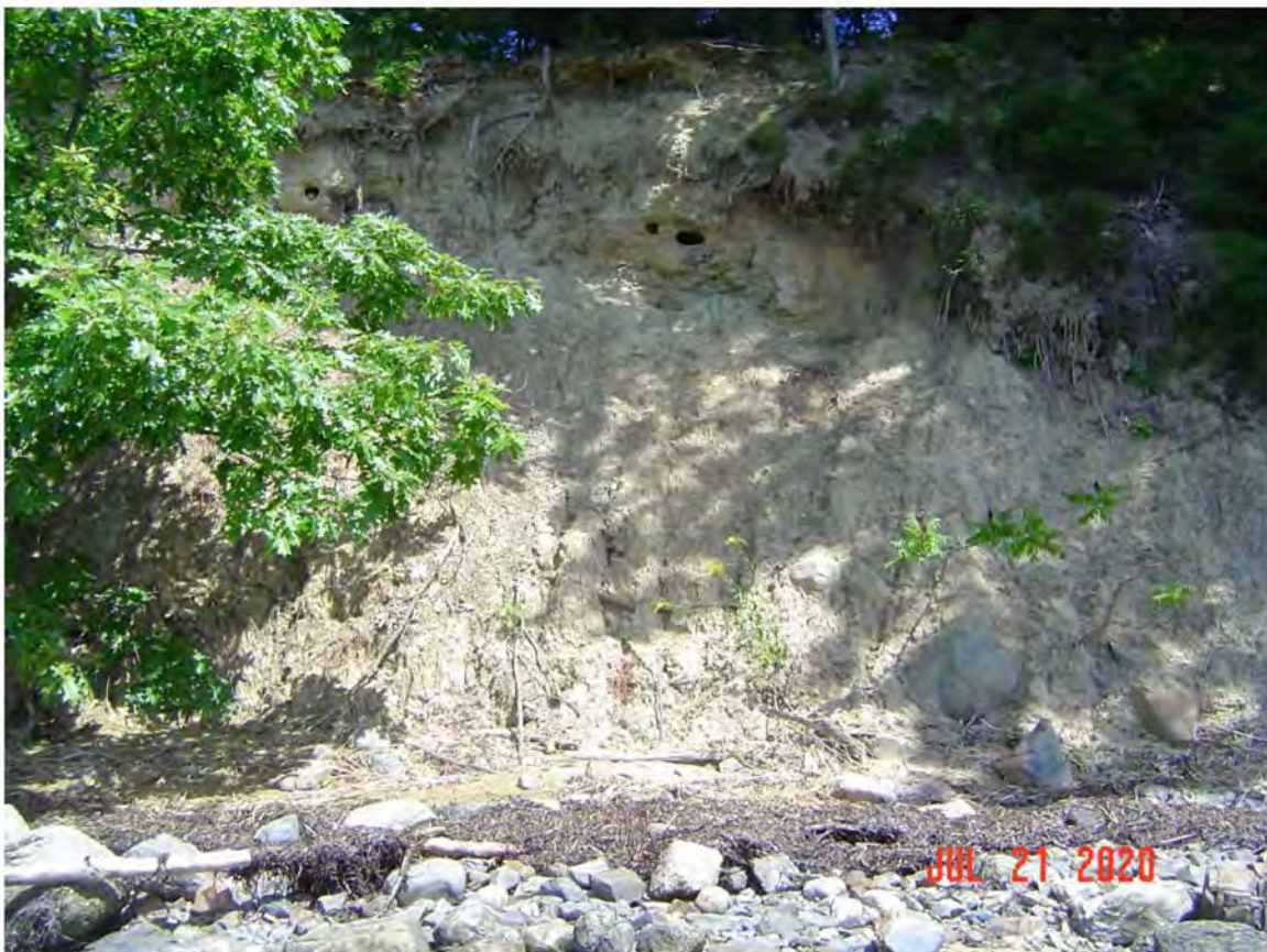
Image 12 – Looking north at low tide at the south side of Fox Point in Newington. Note the severe bank erosion. The distance from the wrack line at the bottom of the image to the top of the bank is approximately 20+ feet. Note the bird nesting cavities near the top of the bank. (©Jacobs2020)
