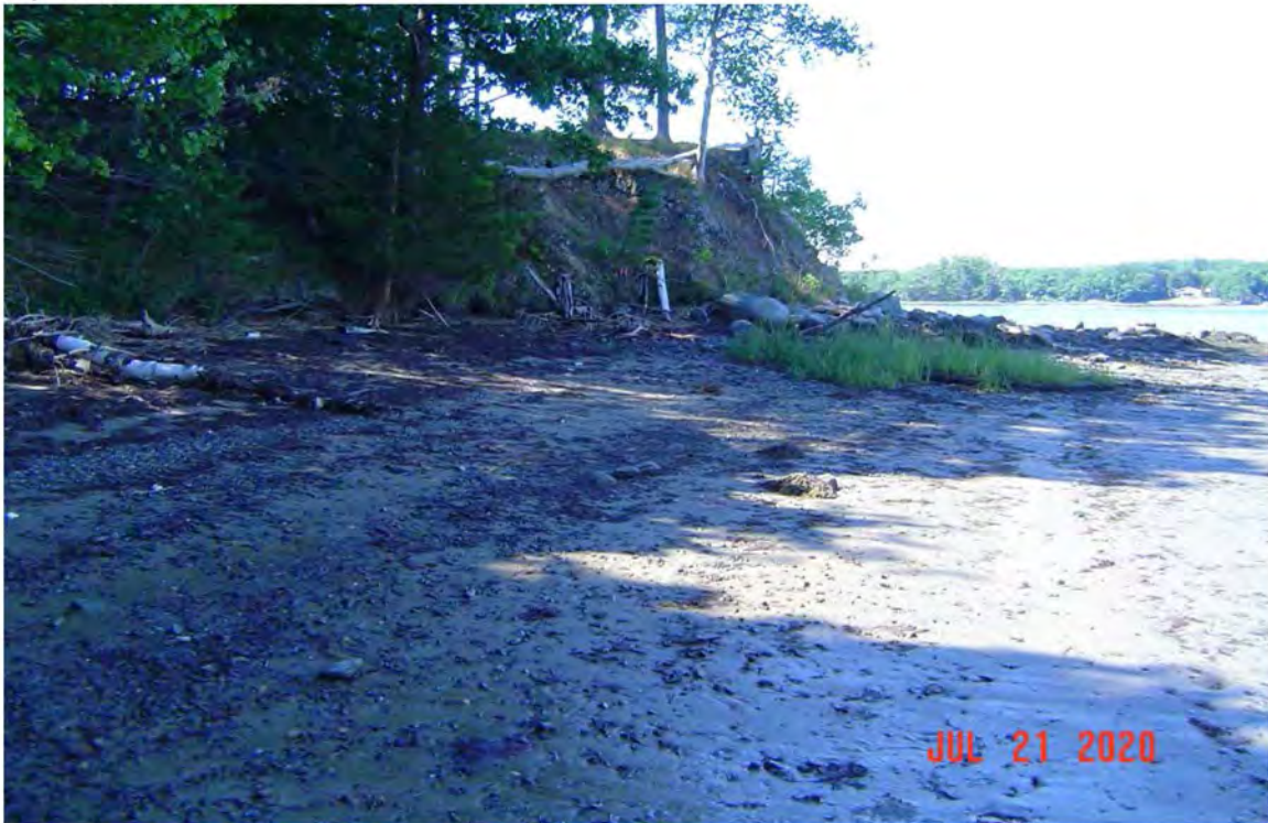
Image 9 – Looking south at low tide from atop the existing water line (and the location in image 7 above) in Newington. Note Fox Point and the severe bank erosion as well as salt marsh. (©Jacobs2020)
