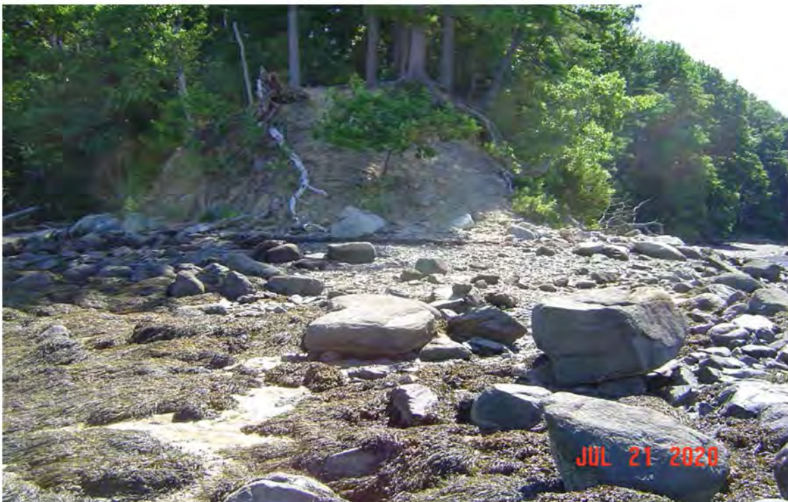
Image 10 – Looking east at low tide toward Fox Point in Newington. Note the severe bank erosion. (©Jacobs2020)
