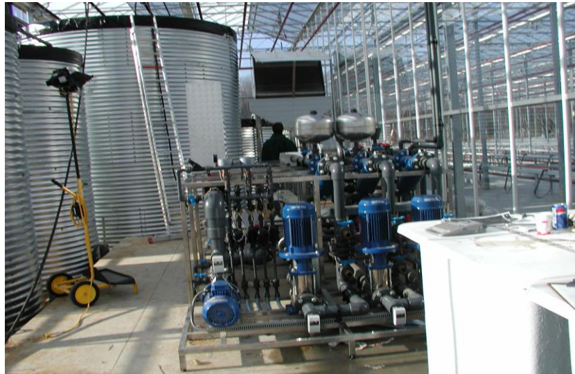
Photo 4. Computerized pumping system with storage tanks and filter
