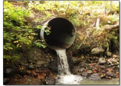
Figure 2 - This undersized metal pipe has caused severe downstream scour and erosion, causing the outlet to become perched above the stream. The crossing overtops, is vulnerable to failure, and is a barrier to aquatic organism passage.
