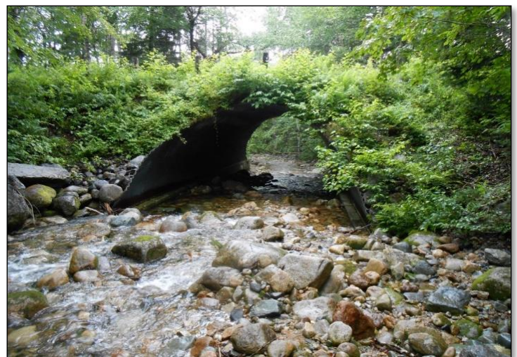
Figure 3 - An open-bottom arch with stream simulation design will accommodate flows during flood events, and maintain full aquatic organism passage and water and sediment transport.
