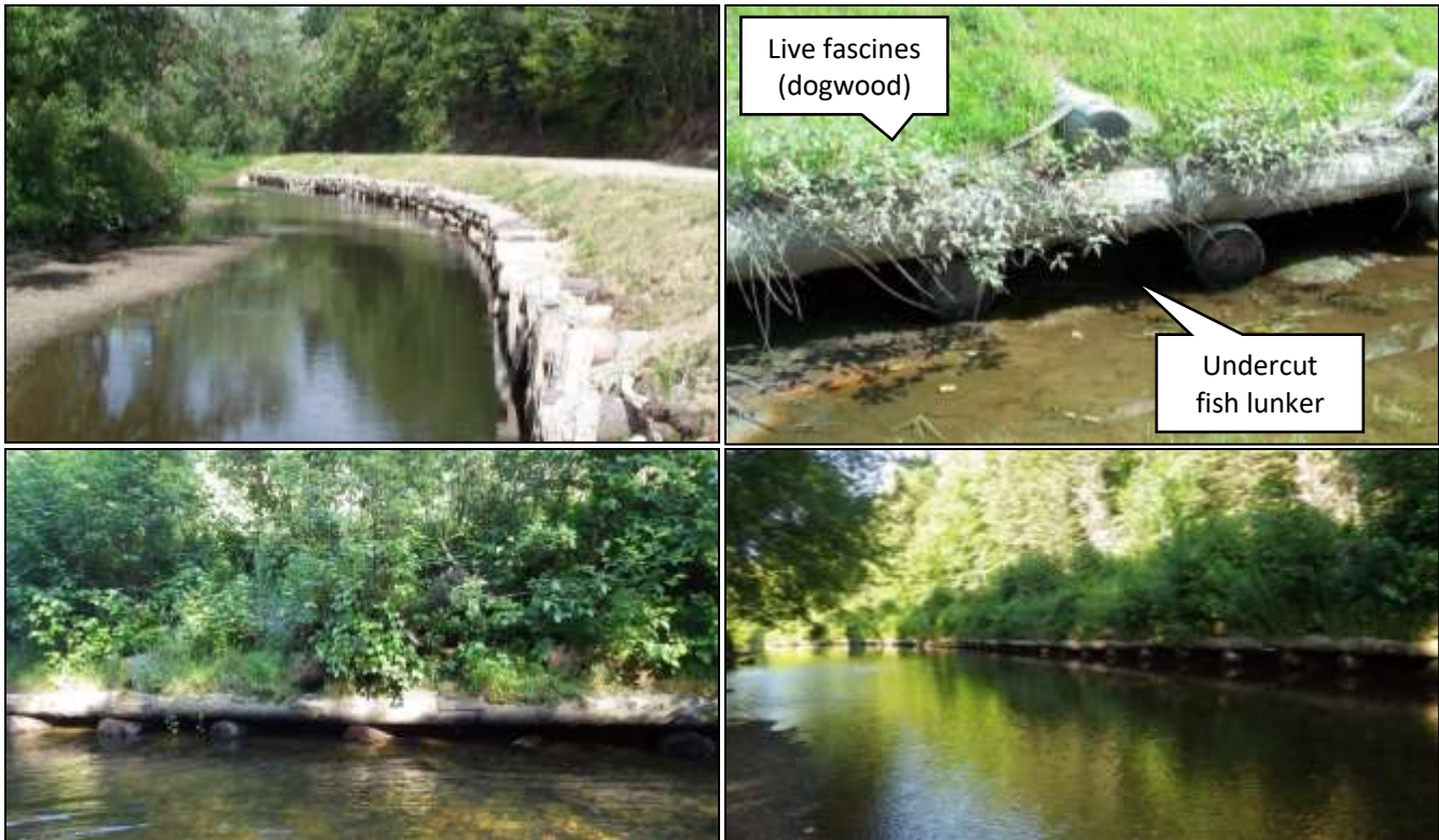
Figure 1 – Example of a successful bioengineered bank stabilization project. These pictures were taken post-construction (top pictures taken in September 2000; bottom pictures taken in August 2017). Live dogwood fascines (bundles of live plants) were used in this stabilization project, in combination with logs and other techniques. The design created a shady area above the water, which benefits native brook trout, a cold-water species known to inhabit this stream.
