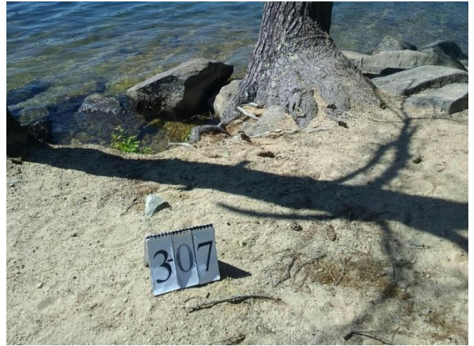
Significant undercutting and erosion at Sandwich Town Beach.
