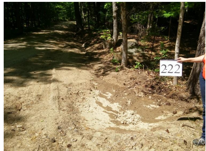
Coolidge Farm Rd steep grades transport significant amounts of eroded ditch sediment to streams.
