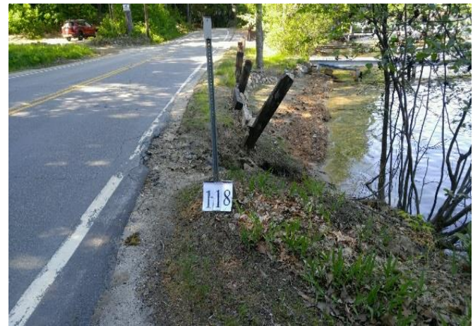
Rt. 113 along Cotton Cove suffers from complex runoff issues.
