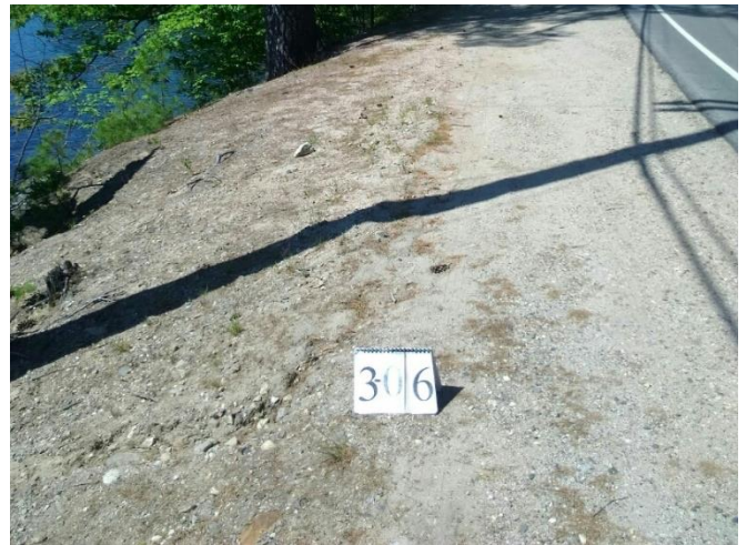
Erosion and poor buffer at Squam Lake Rd pull-off area.
