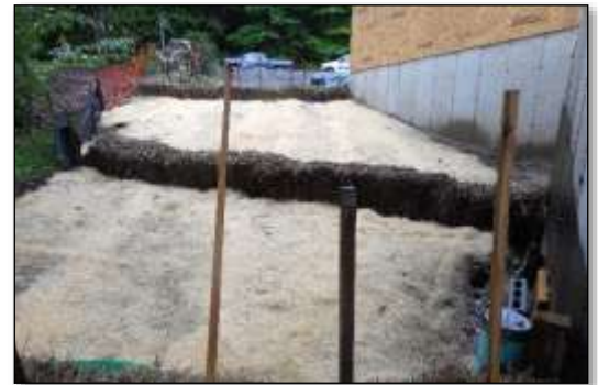
Figure 2 - Hay bales and biodegradable erosion control matting minimize erosion on this slope.
