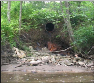
Figure 4. A Stormwater Outfall Discharging Untreated Runoff to a Stream (Photo: FB Environmental)
