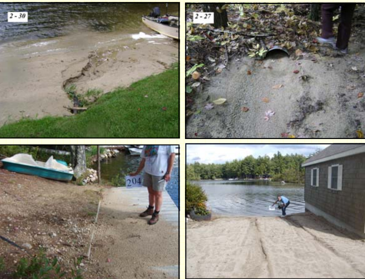
Examples of Identified Erosion Problems
