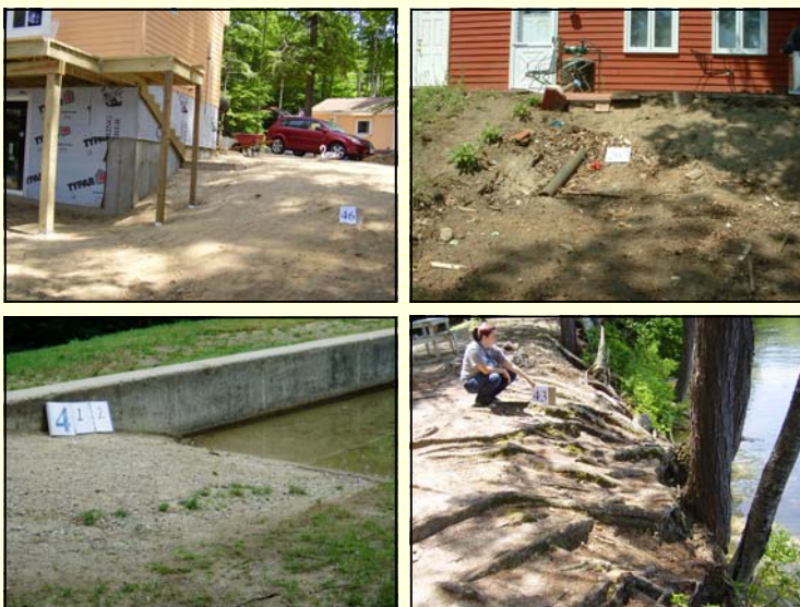
Examples of Identified Erosion Problems
