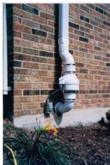
Typical vent fan (EPA 2012)
