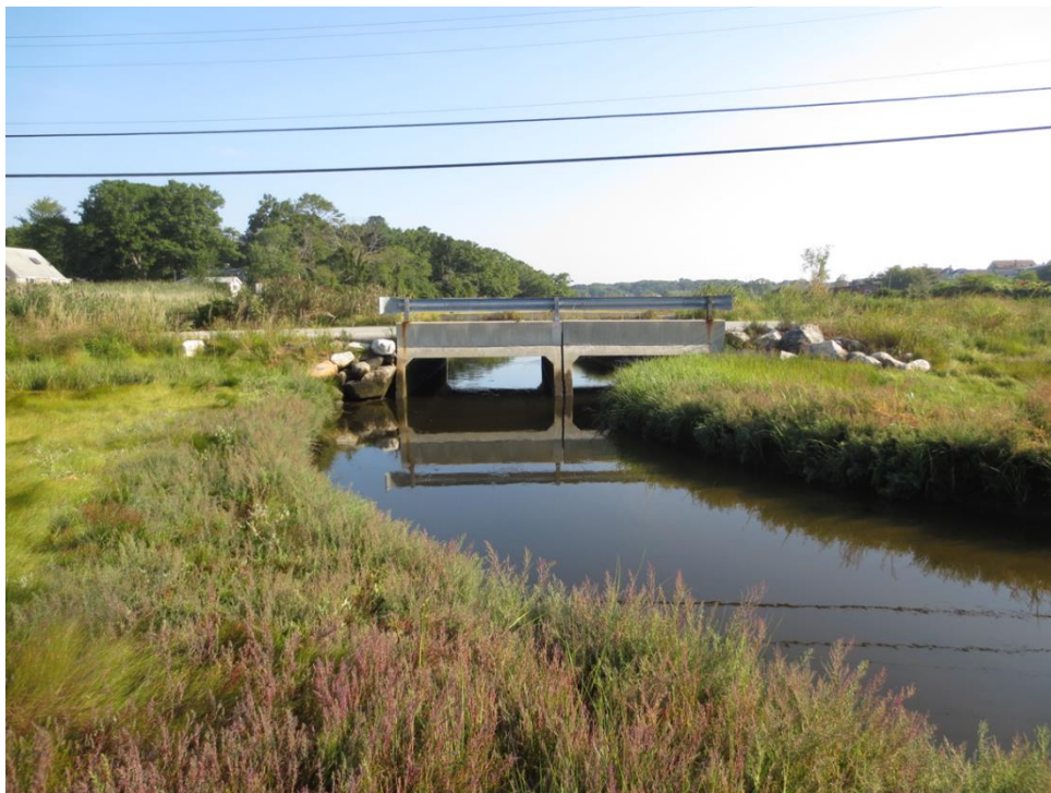
Figure 22. Crossing 54 at Parsons Creek and Wallis Road is a restoration site that received good scores for tidal range, vegetation, salt marsh migration; however, the road is very low in elevation and subject to periodic inundation and thus received high inundation risk scores.
