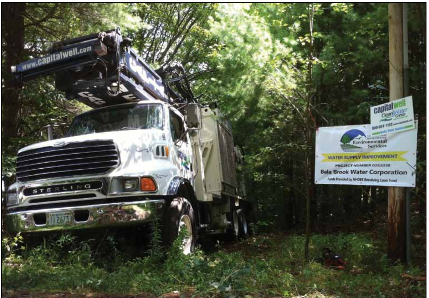
Well drilling rig getting positioned between some trees. The new well was drilled to approximately 800 feet, with a preliminary yield of 10 gallons per minute.
