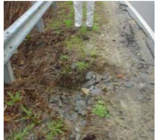
Road erosion into the stream near BCH24.
