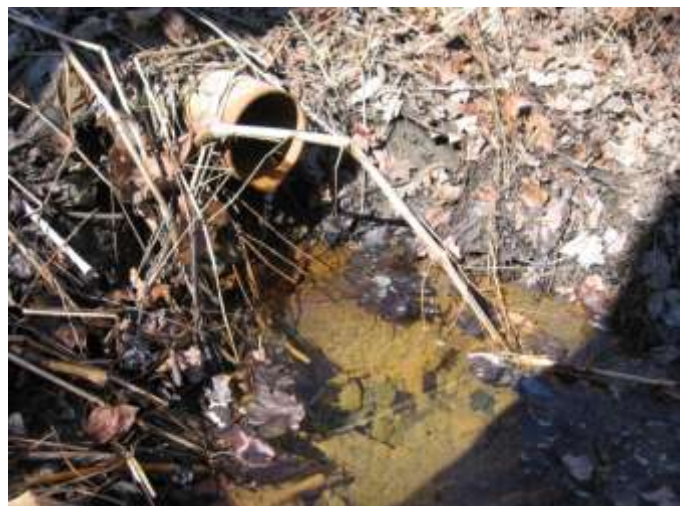
Pipe discharge in a wooded area near site BCH 18.
