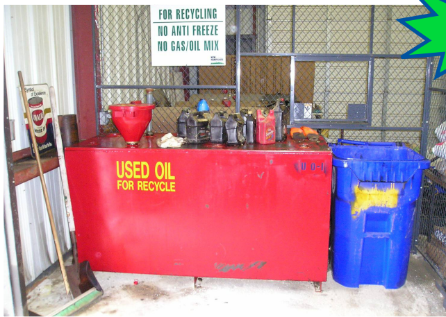
Tank is indoors, on a concrete surface and is correctly labeled. Customers leave oil jugs on top of tank for facility operator to inspect and empty into tank.
