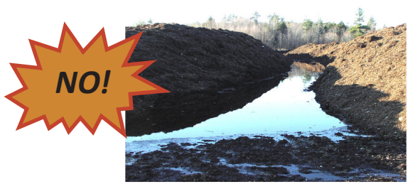
Compost piles are too close to one another and too tall. Poor drainage is allowing water to accumulate between windrows.
