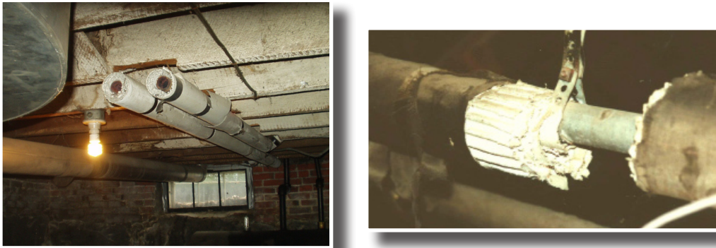
Figure 2: Friable pipe insulation
