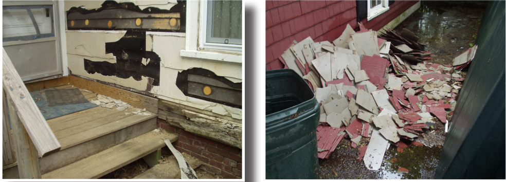
Figure 1: Non-friable asbestos shingles
