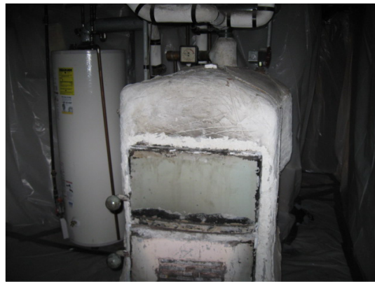
Figure 3: Friable asbestos insulation on an old furnace
