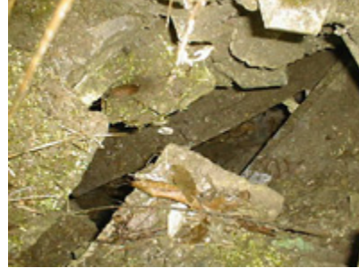
Layers of buried asbestos board waste viewed through hole in the ground
