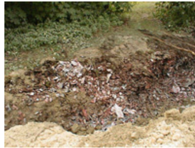
A mix of red, white, and grey asbestos sheet scrap uncovered while excavating a trench
