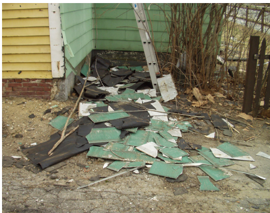
Improperly removed asbestos from home renovation project.
