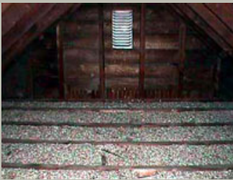
Vermiculite insulation found in an attic.
